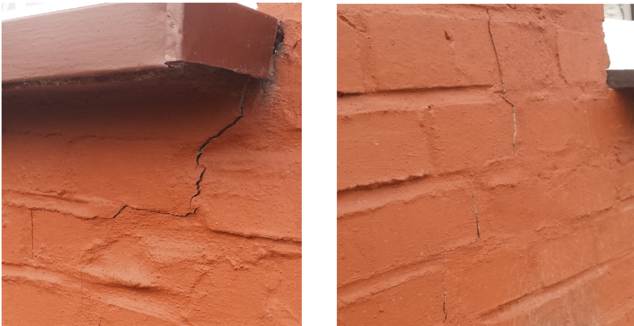
Photo 6. Technical condition of the monitored building after the exploitation front passed, September 2015 (Source: own elaboration)
