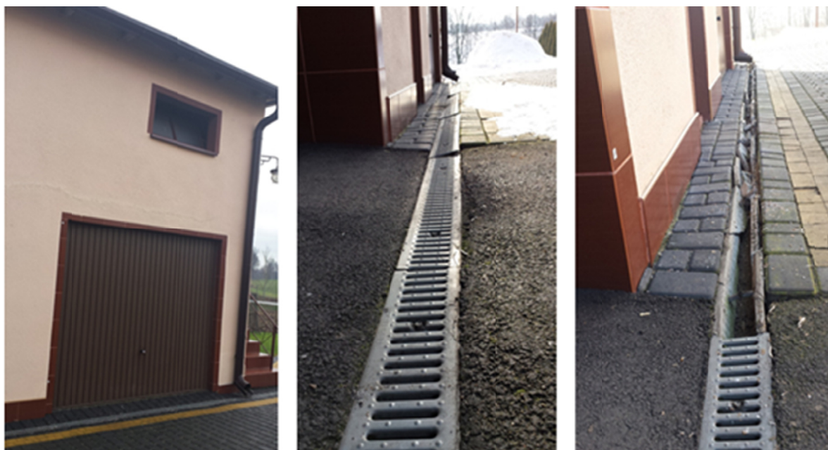
Photo 4. Damage to the drainage trough at building No. 4g, which increases in time (Source: own elaboration)
