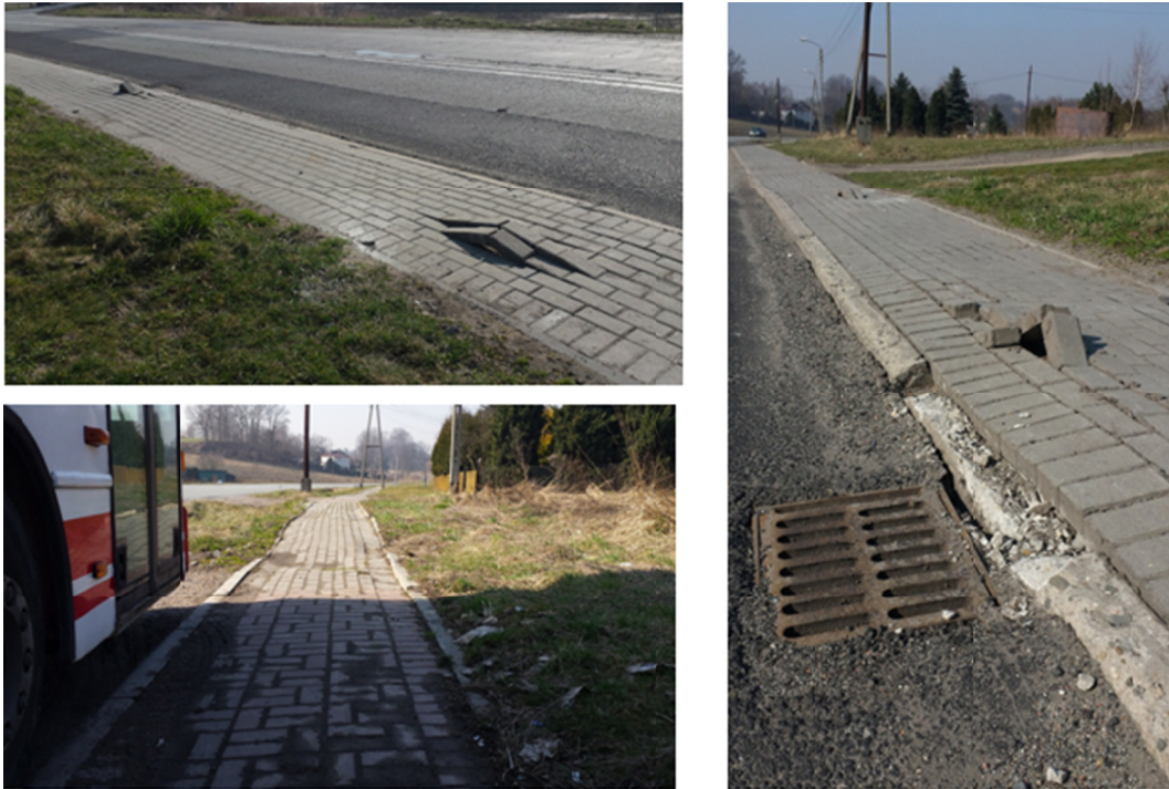
Photo 5. Pavement surface damage at the main street in Marklowice (Source: own elaboration)
